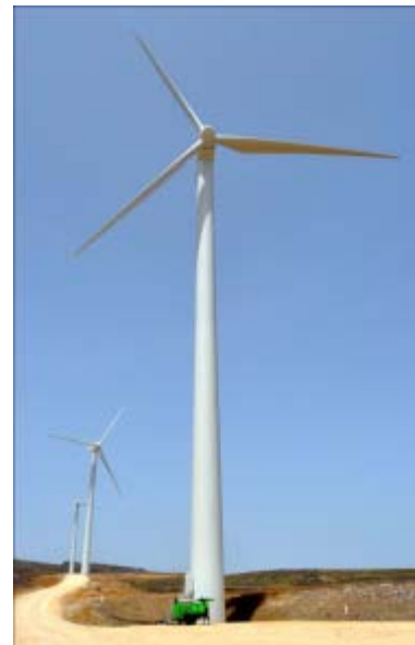
8 MW Wind Farm, in Sal, Cape Verde Commissioned in March 2012
