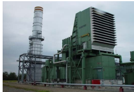
Machala Power Thermal Power Plant
