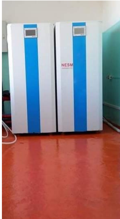
System control room after
