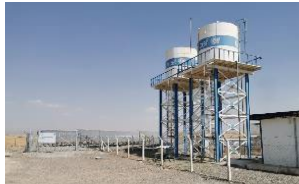
A solar plant installed at a borehole in Darashakran refugee camp (Iraq)
