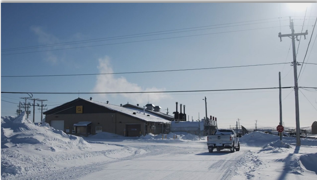
Diesel generating station in KUUJJUARAAPIK, Nunavik, Québec
