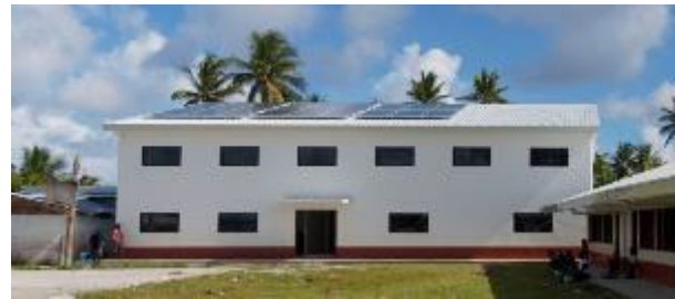
School in Chuuk using standalone solar PV with battery storage
