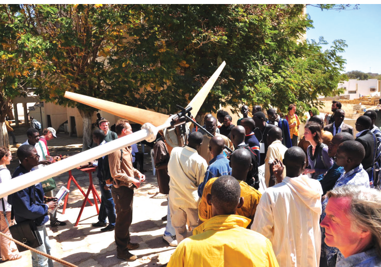
Image 7 Installation of a small wind turbine at the University of Dakar ©www.eolsenegal.com
