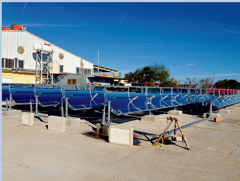
Photograph: Inventive Power A.S.
