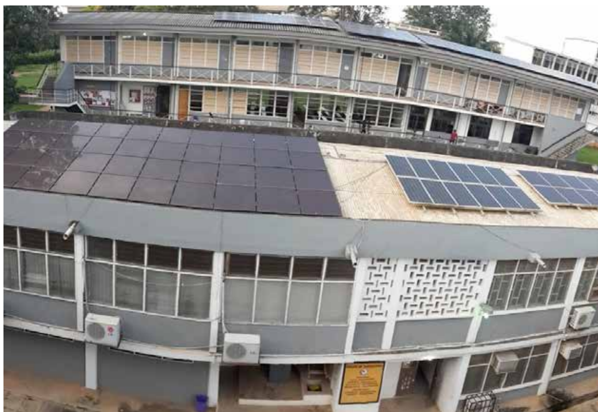
A section of the solar PV panels of KNUST's 24 kWp system Photo: Ministry of Power
