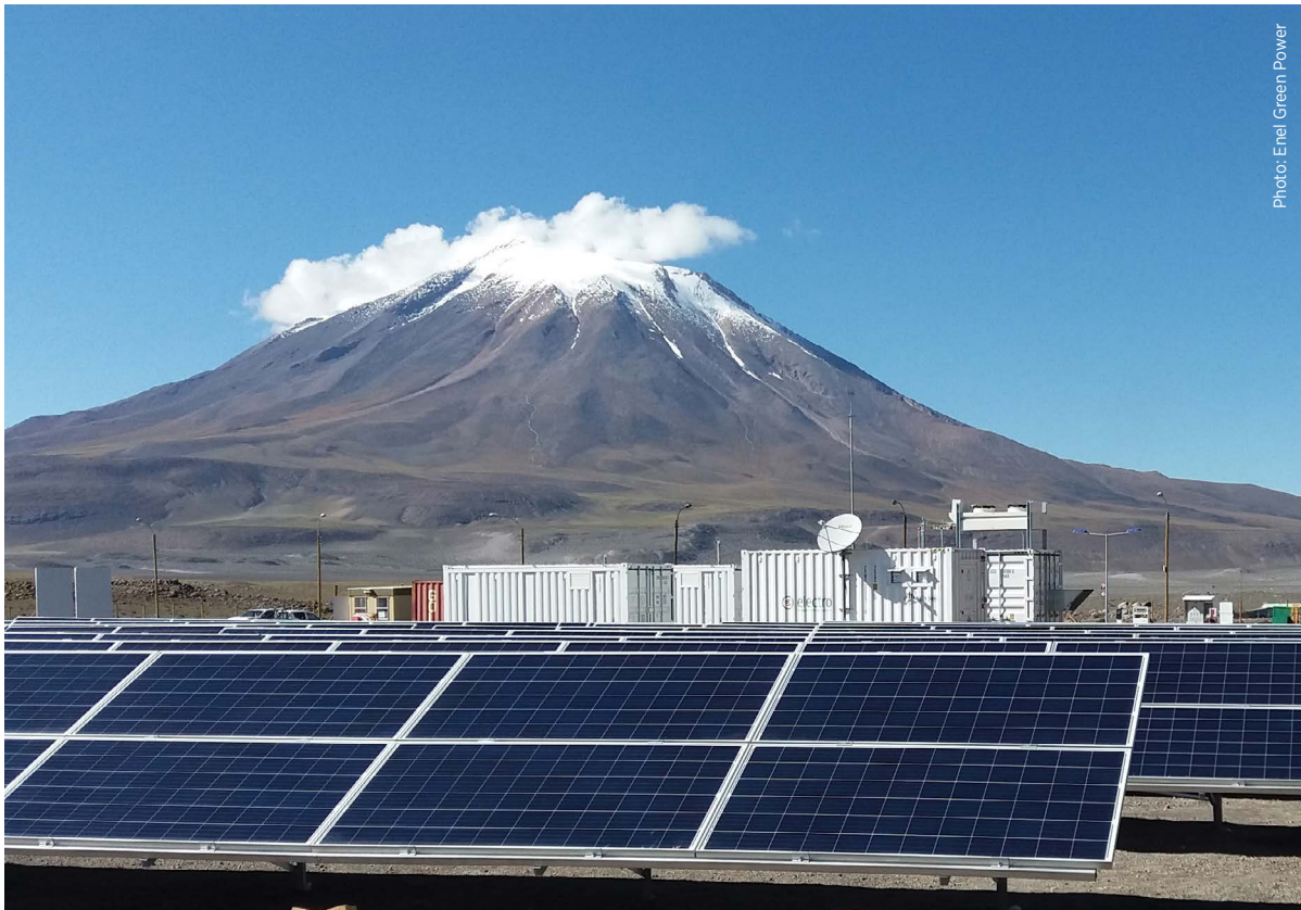
Electrolysers installed by Enel Green Power in 2017 in the geothermal Cerro Pabellón plant. The electrolysers are part of a micro-grid solar PV facility combined with two energy storage systems, one based on green hydrogen.
