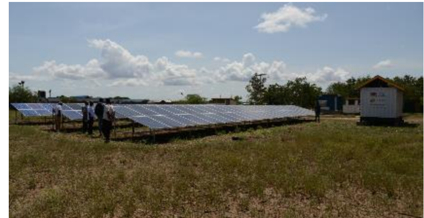
Standalone solar system with containerised battery bank
