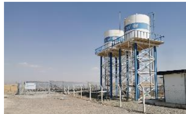
A solar plant installed at a borehole in Darashakran refugee camp (Iraq)
